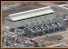
Phase 2 Boil-off gas compressors
