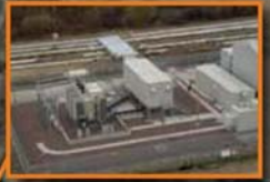
Phase 2 132kV to 11kV substation
