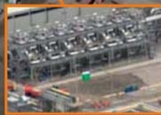
Phase 2 Ex-tank pumps
